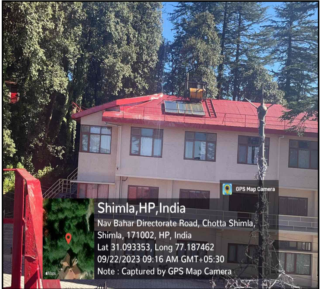
Solar Water Heater
